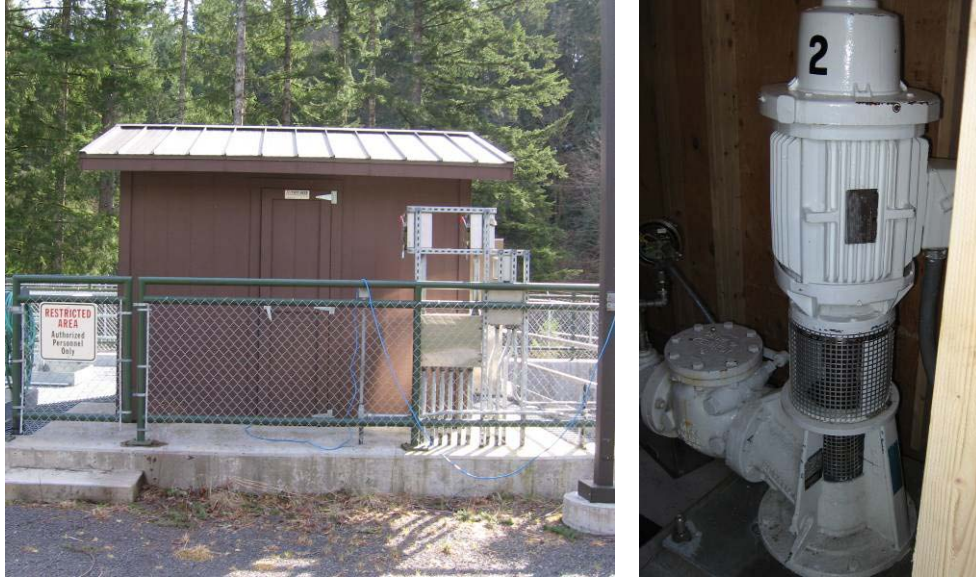
Pumps feeding Elevated Water Tank (one of two pumps shown)
