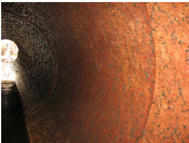
Non-chlorinated section of pipe at Landsburg; periwinkle growth after one year
