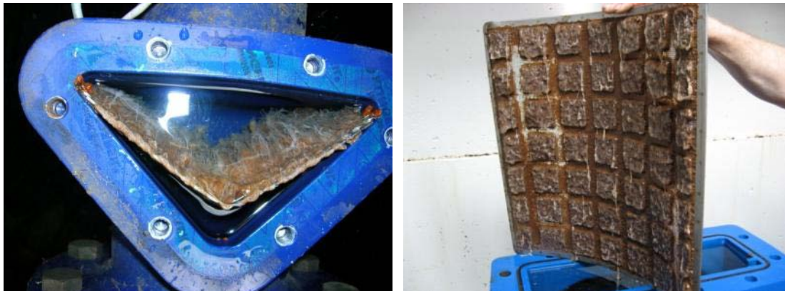
Algae Growth Clogging Downstream Facilities (left photo = wholesale meter screen; right photo: strainer for pressure reducing valve)
