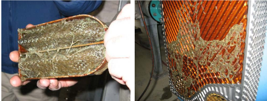
Algae Growth Clogging the Cedar Treatment Facility in 2008
